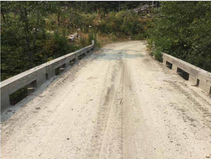
Sediment on deck at right approach
